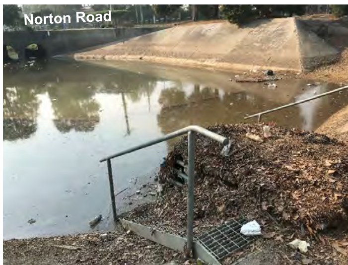
Figure 2-8 Blockage of sedimentation pond outlet pit at Melbourne Water’s Croydon Main Drain
